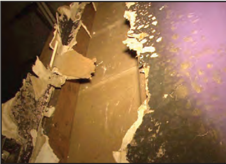
Fire crept up the wall of the youth room, inches from the ceiling.
