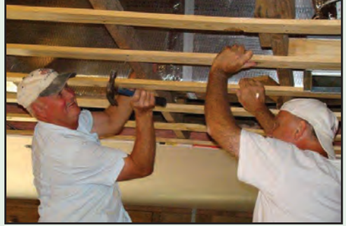
Clarence Littlefield hammers a ceiling panel in place during a mission project in Buras, La.
